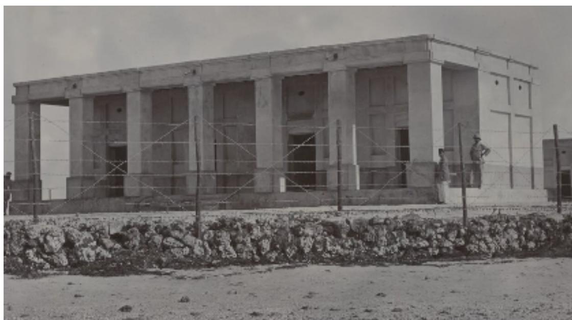
Figure 2 One of the newly constructed buildings in the quarantine site at Bu Maher (8)
