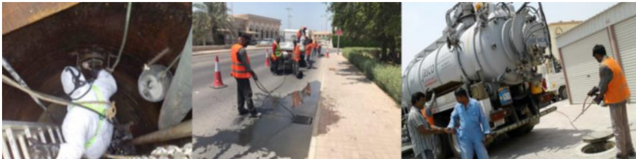
Suction tanks used during emergency situations
